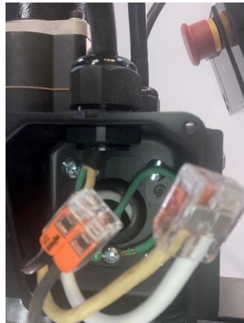
Fig. B. Installed Wiring
