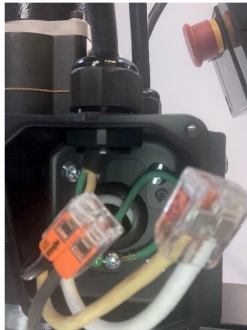
Fig. B. Installed Wiring
